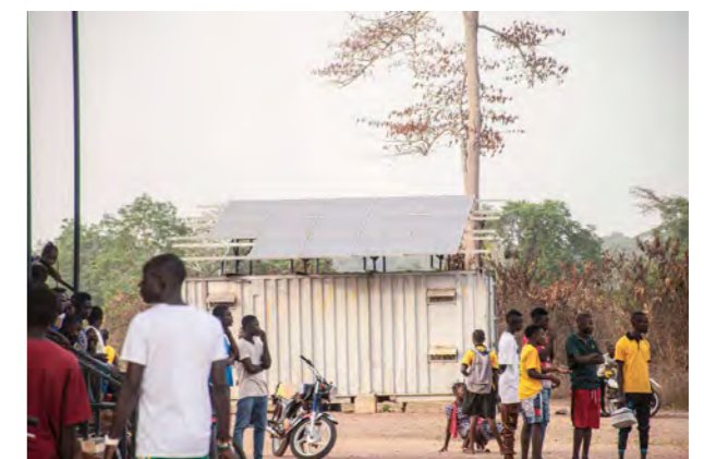
Solar electrification system
