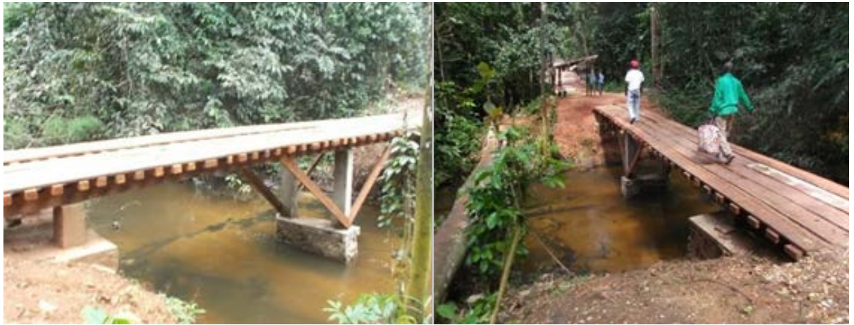
Mongambé Bridge rebuilt to facilitate access to strategic tourist sites in the APDS. ©APDS
